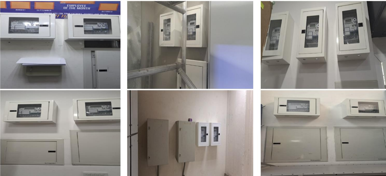
Prepaid energy meter Work status
